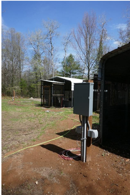
New electrical box with multiple possibilities.
